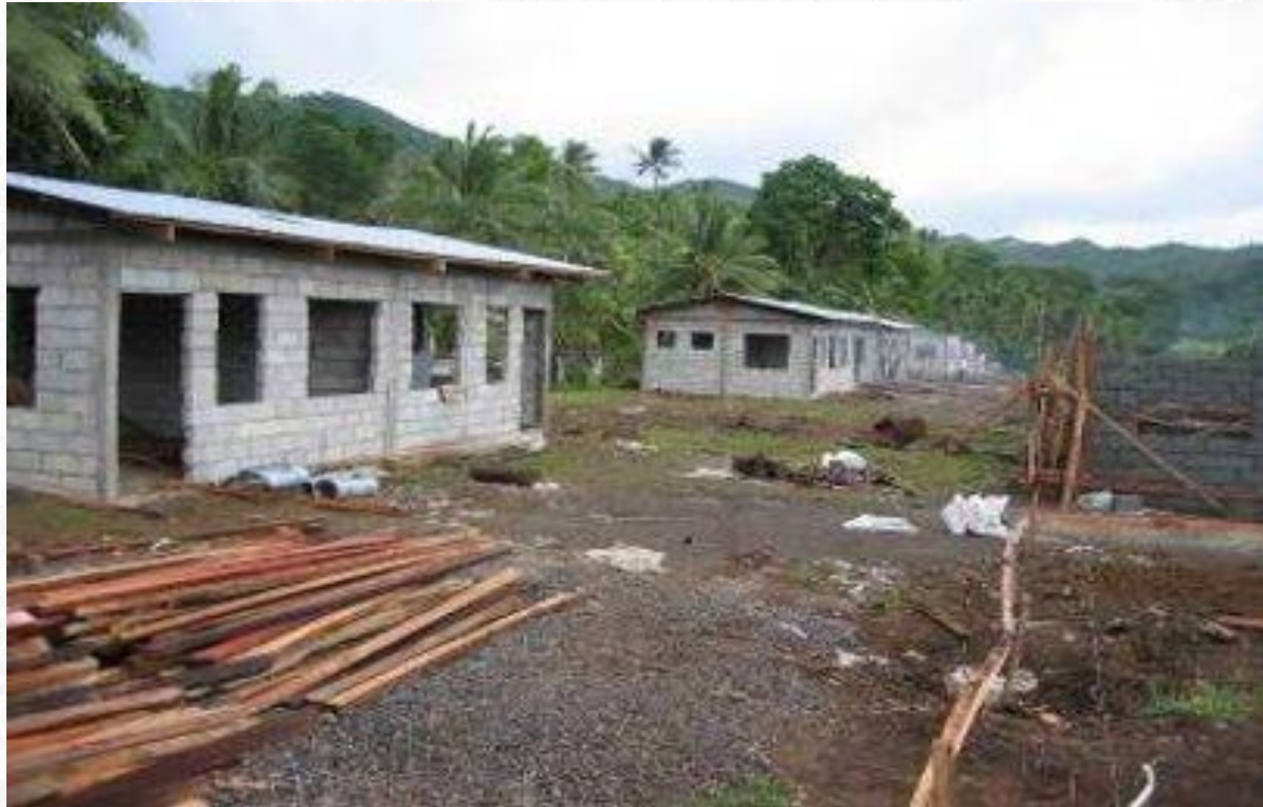
Support rebuilding of shelters on higher/ safer ground in flood prone areas
